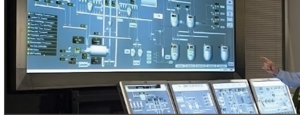
Building Management System
