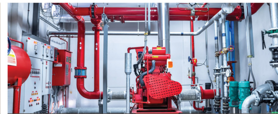
Fire Control System
